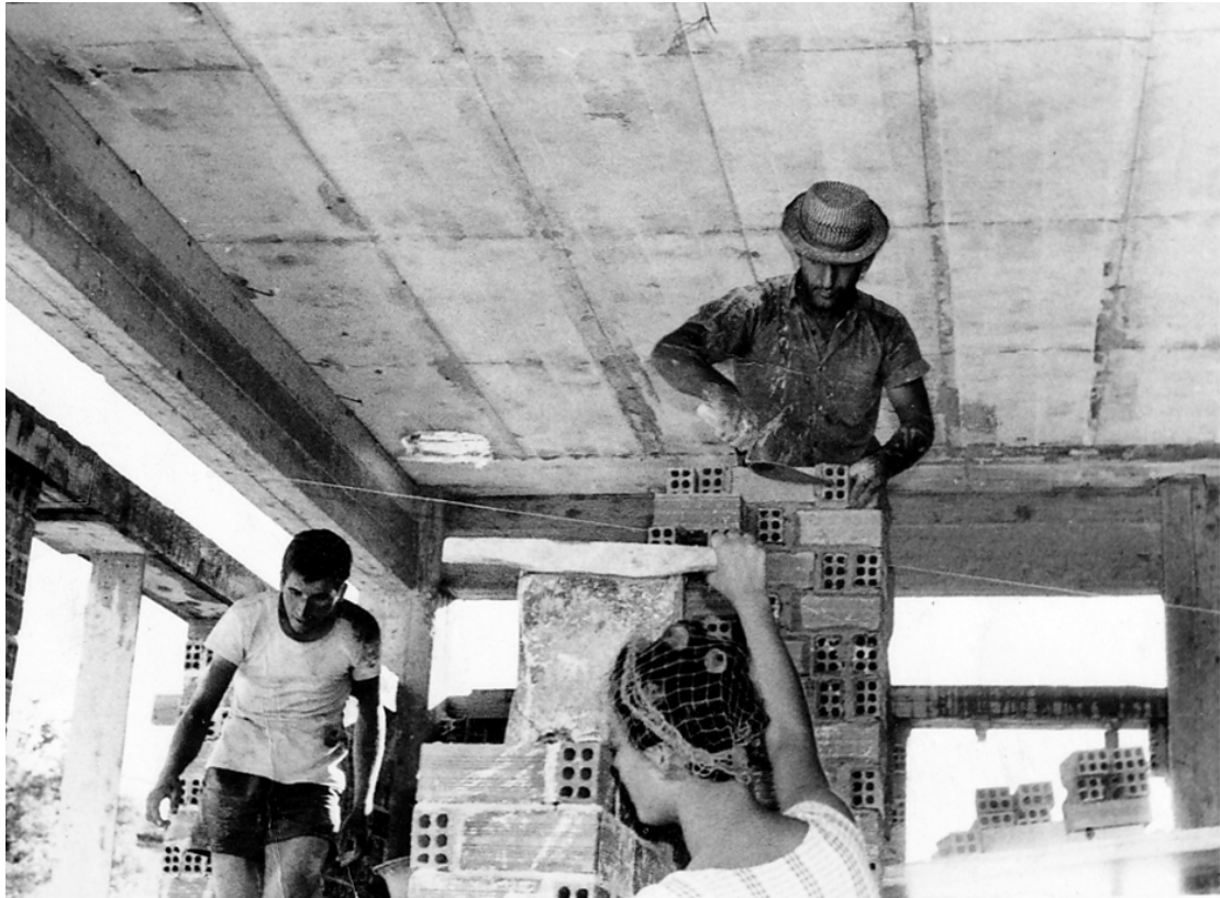
Building the modern Athenian apartment (1960s, photo credits: D. Koutroumpilas personal archive)
